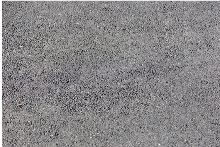
Figure 10. Pavement showing light raveling
