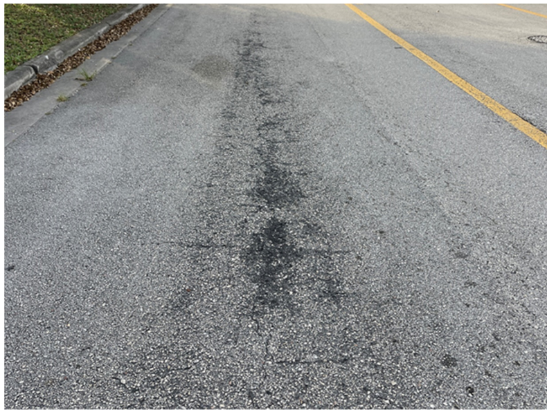
Figure 9. Pavement showing moderate raveling
