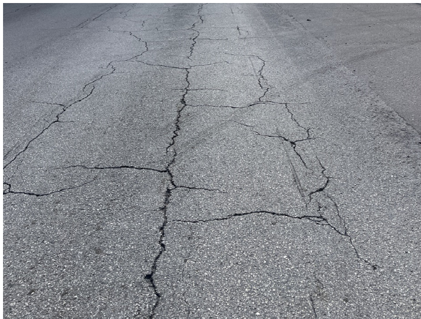
Figure 3. Class III crack, extend in a longitudinal direction
