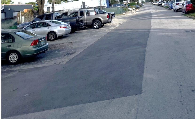
Figure 11. Longitudinal patching on pavement
