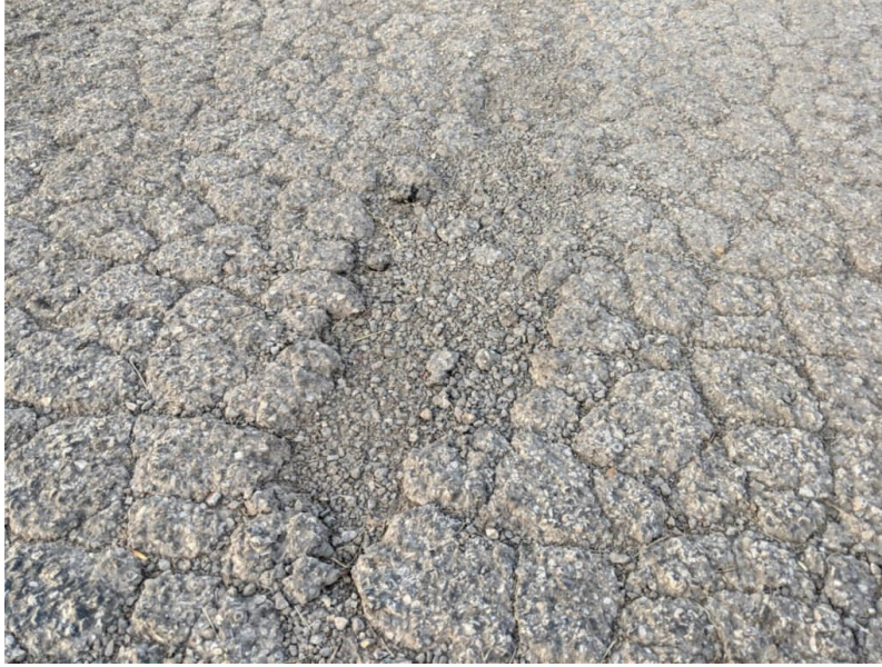
Figure 8. Pavement showing severe raveling
