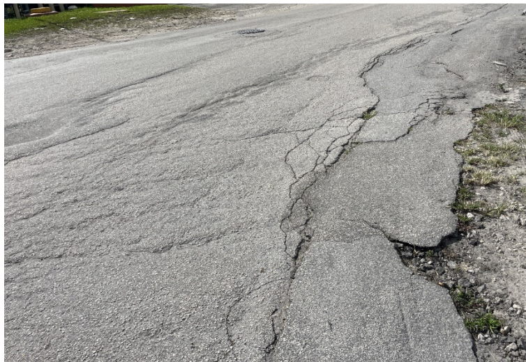
Figure 7. Advanced rutting with severe pavement displacement
