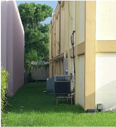
Repetitive Loss Area 4 - Elevated HVAC unit
