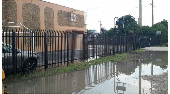
Repetitive Loss Area 3 - Water ponded in parking lot
