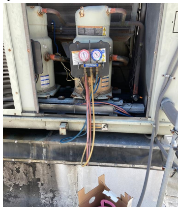
Figure 1 Existing situation of leaking unit with the replacement refrigerant on floor
